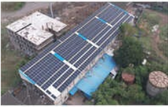
250 KW Trunkey Project
