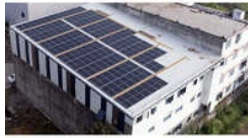
70 KW Trunkey Project
