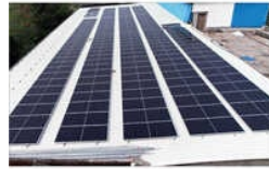
200 KW Trunkey Project
