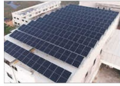
100 KW Trunkey Project
