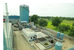
Effluent Treatment Plant
