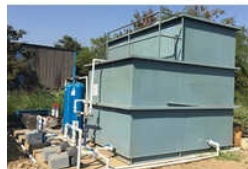
Packaged Sewage Treatment Plant
