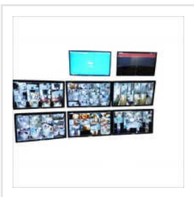
CCTV Control Room
