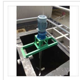
Industrial Wastewater Aerator
