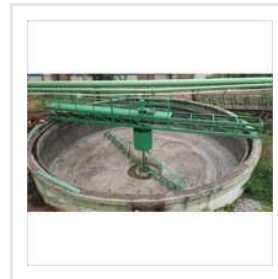
Industrial Wastewater Clarifier
