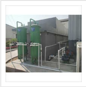
Industrial Effluent Treatment Plant
