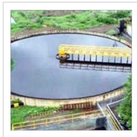
Incline Plate Clarifier
