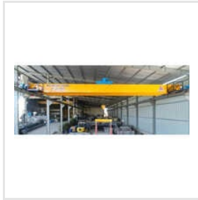
10 Ton Single Girder EOT Crane
