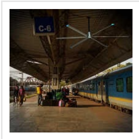
Railway Platform HVLS Fans
