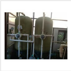
Commercial Water Softener With Filtration
