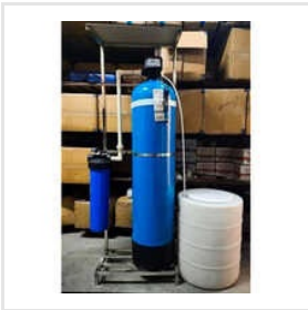
1000 LPH Water Treatment Plant With
