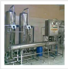
5000 LPH SS RO Plant
