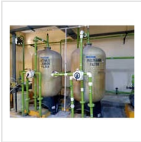
30000 LPH Water Treatment Plant With
