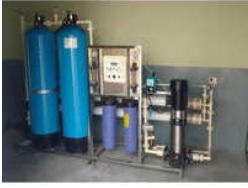
Industrial RO Plant Installation Service
