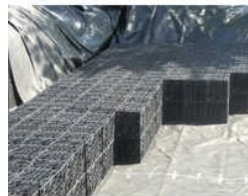
Industrial Rainwater Harvesting System
