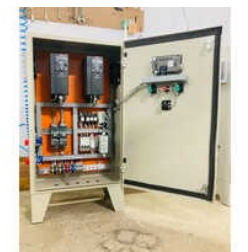
Mild Steel VFD Panel
