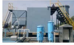
Industrial Effluent Treatment Plant
