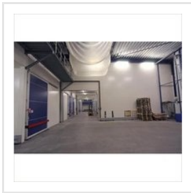
Control Atmosphere Cold Storage
