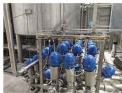
Industrial Valve Cluster
