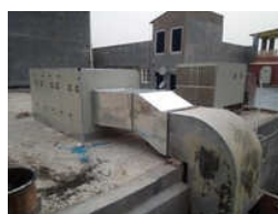
Kitchen Exhaust Scrubber
