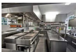
Restaurant Kitchen Equipment
