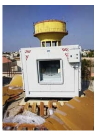
DRI Evaporator Evaporative Coolers
