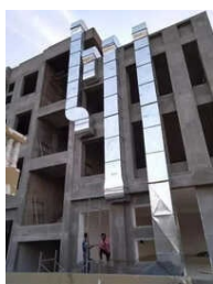
Galvanized Iron Kitchen Exhaust
