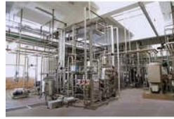
Stainless Steel Milk Processing Plant
