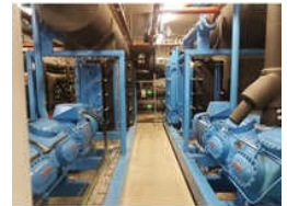
Industrial Ammonia Refrigeration System
