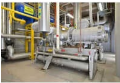
Ammonia Cooling Refrigeration System
