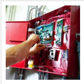
Fire Alarm Systems Maintenance Service
