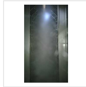
PT Line Spray Zone
