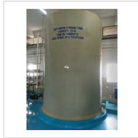
Soft Water Storage Tank
