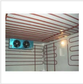
Electric Cold Room
