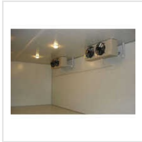
Cold Storage Plant
