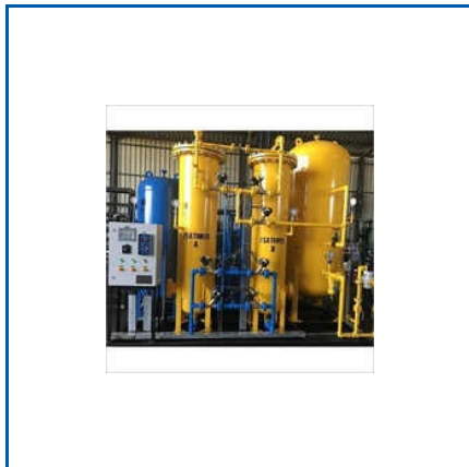
INDUSTRIAL NITROGEN PLANT
